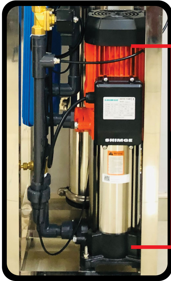
Reverse Osmosis Pump (P-1)
