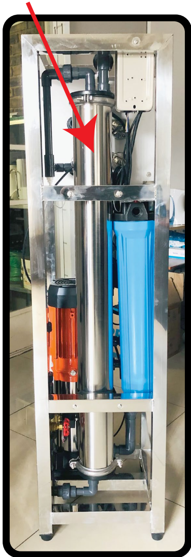
Reverse Osmosis Vessel (RO-1)
