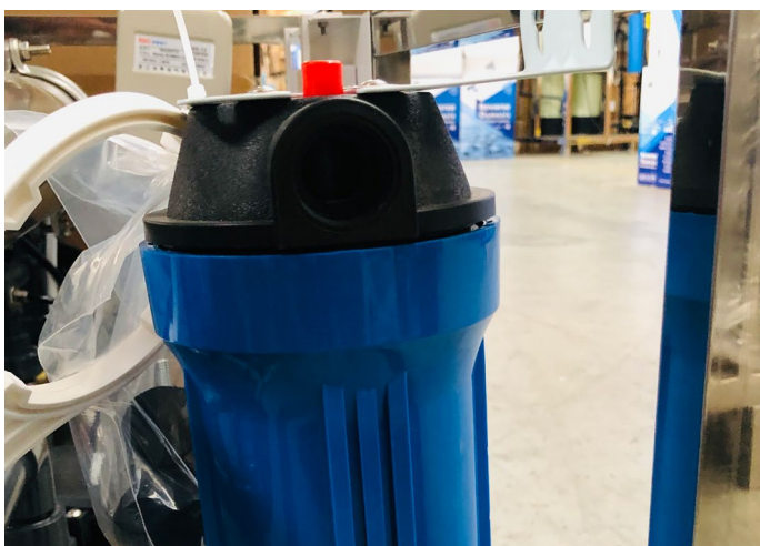
A: Feed water inlet connection, from the 20" blue filter .
